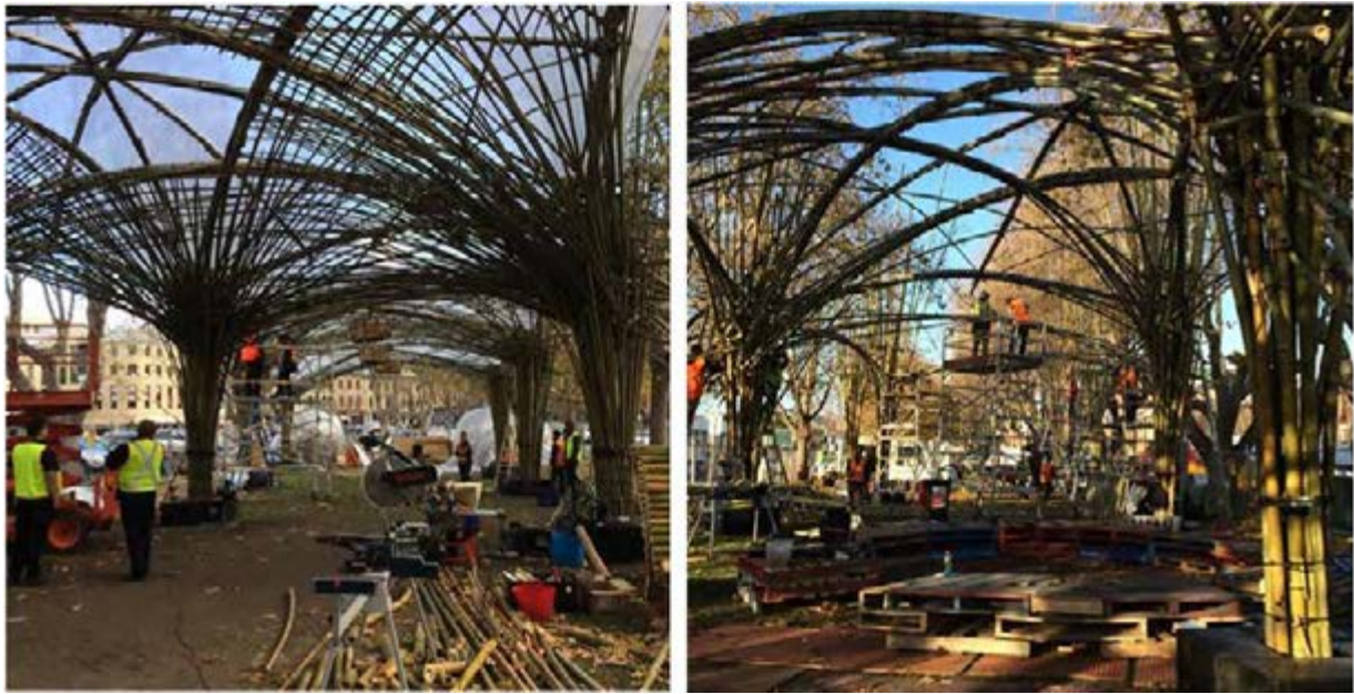
Figure 4: Roofing complete on central bay (left) and end bay (right). Images: Helen Norrie.
